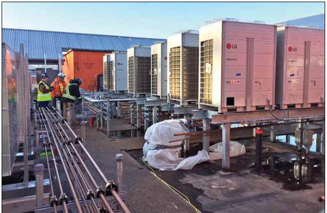
Outdoor units and refrigerant piping for the Southport VRF system.
